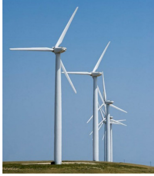
Figure 3: Utility scale wind turbines at the Cedar Creek Wind Farm in Grover, Colorado. Photo by Dennis Schroeder / NREL.
