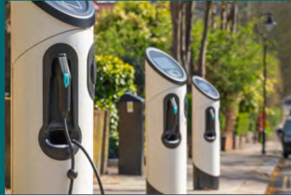
Figure 1: EV charging stations
