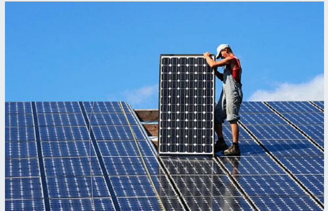
Figure 3: SPV Rooftop Installation. Source
