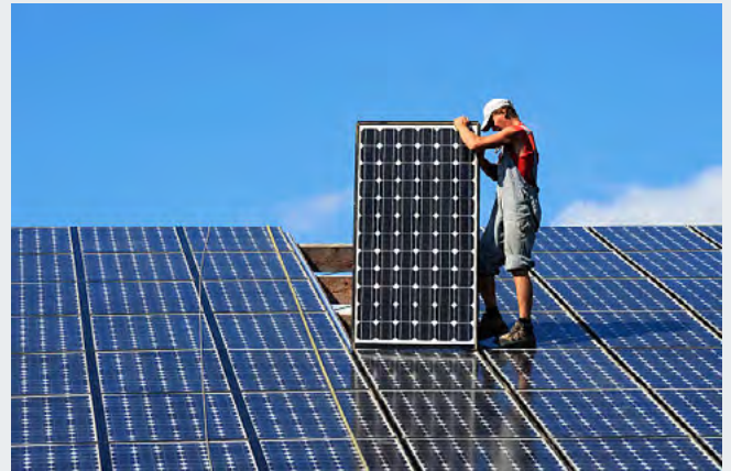
Figure 3: SPV Rooftop Installation. Source
