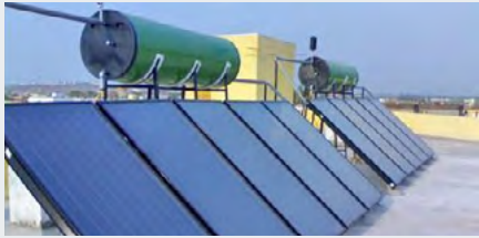
Figure 2: Solar flat plate collectors (FPC)
