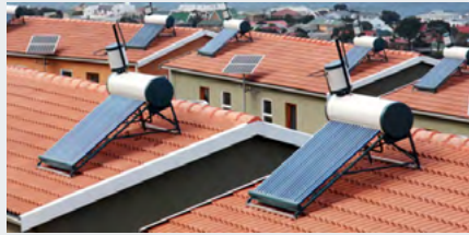
Figure 3: Evacuated tube collector (ETC)
