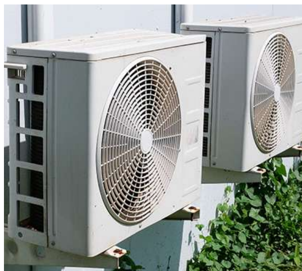
Figure 8: Heat pumps. Source: BC Hydro
