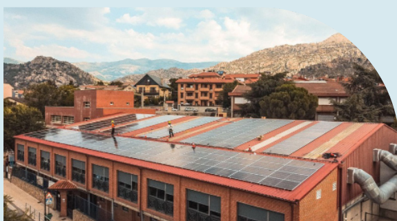
A 100 kWp PV plant adorns the town sports center
