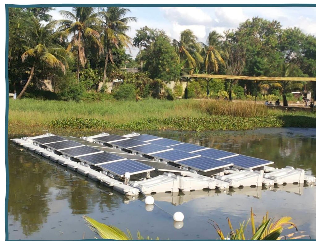
Source: A solar pilot project on a flood control waste pond in Indonesia. Credit: Ciel & Terre International
