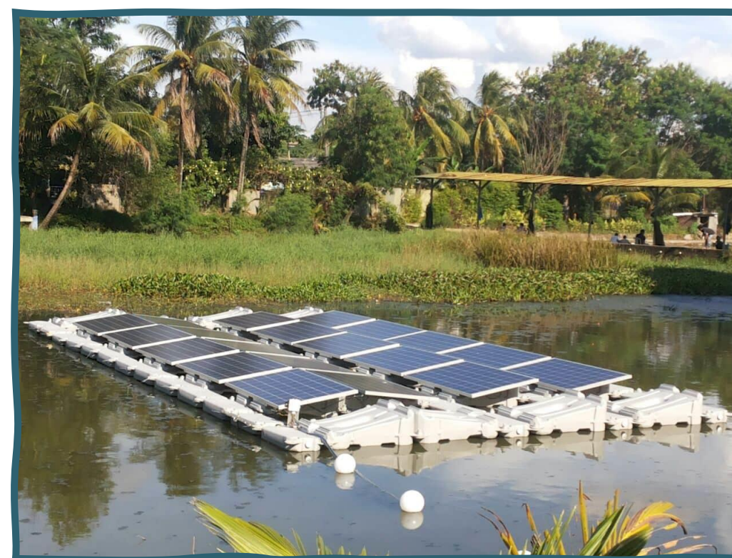
Source: A solar pilot project on a flood control waste pond in Indonesia. Credit: Ciel & Terre International
