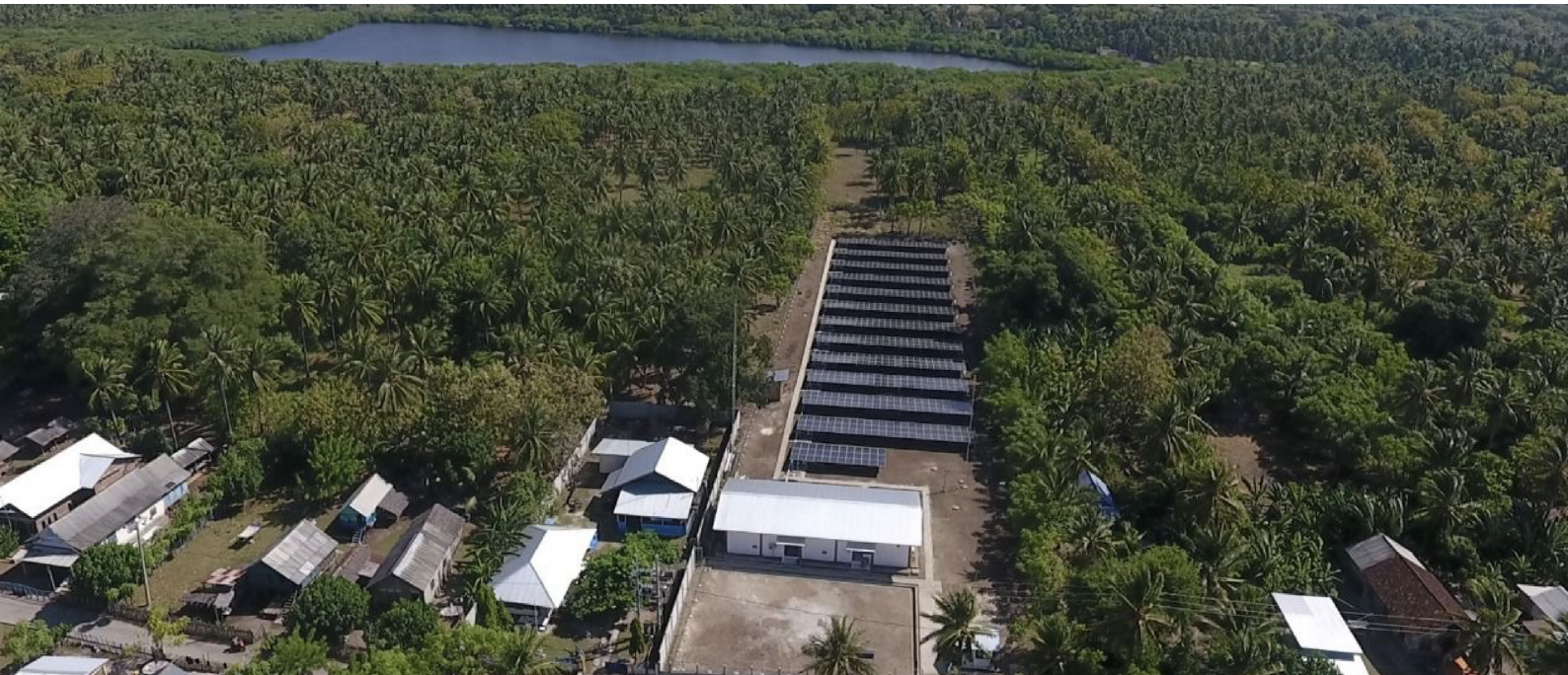
Figure 2. The Solar PV Power Plant on Medang Island, Sumbawa, WNT, has a capacity of 314 kWp and is equipped with a 550 kWh battery and an inverter, supplying 2,574 households on the 4.35 km 2 island with 24-hour electricity (Photo source: PLN)
